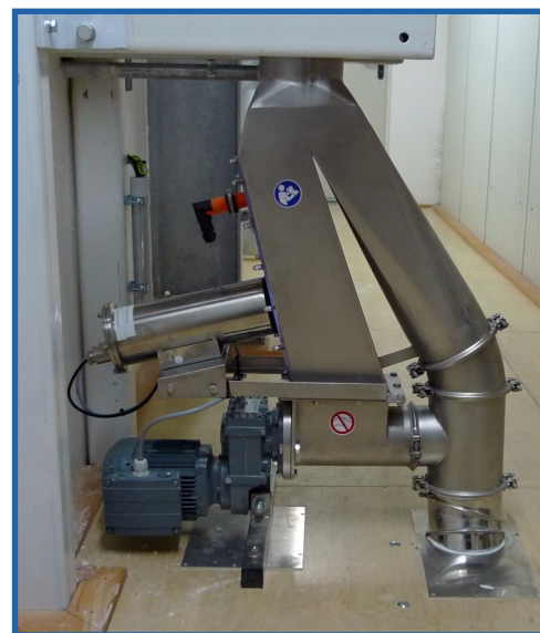
Bypass with camera
